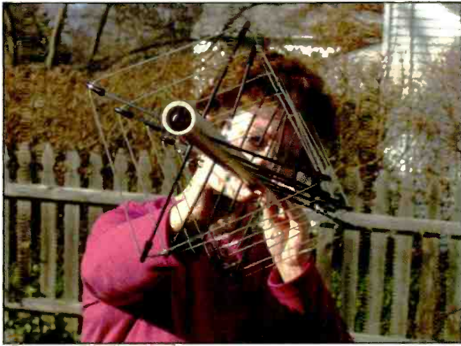
Here's Carolyn giving the Cubex quad the eye! Sighting down the boom helps you properly square the spreaders. (You didn't think I'd be able to get my wife to bolt it to the house while I watched, did you?)
