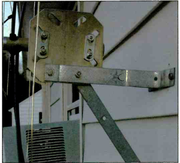
An old galvanneal wall-mount was rigged to hold the Cubex quad in a fixed position against the house.
